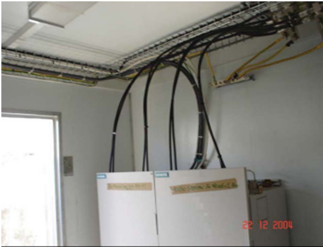
Feeder cable runs in indoor shelter and electrical installations
