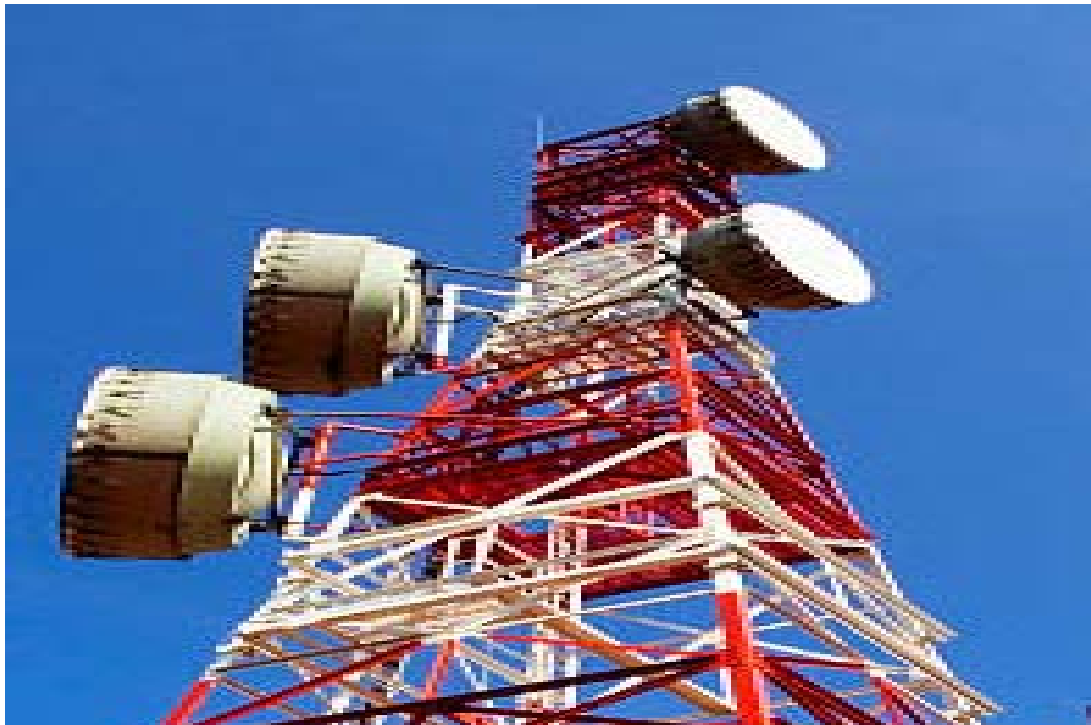
Microwave dish on tower
