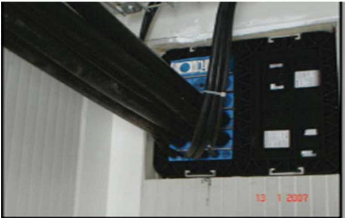
Feeder cables entry to shelter room
